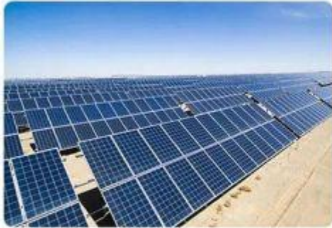
PV power station system
